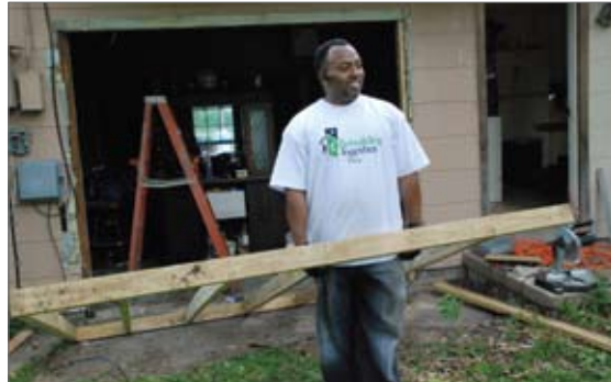
(upper left) Skilled volunteers from All Souls Unitarian Church. (bottom left) Volunteer from Honeywell builds wall where one did not exist. (right) Skilled volunteer from MPW Engineering repairs exterior siding.
